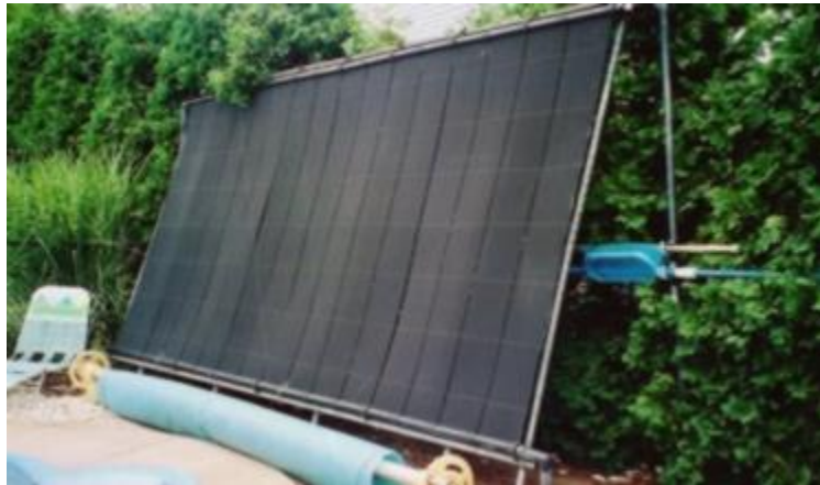
Photo 17-5: DHPE Solar Water Heater
