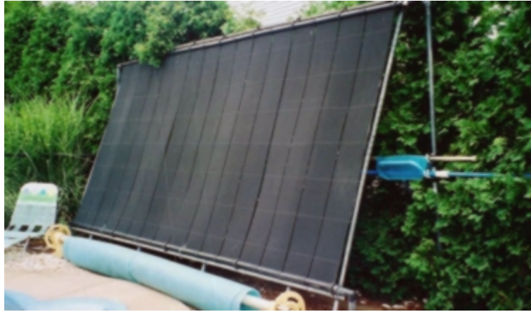
Photo 17-5: DHPE Solar Water Heater
